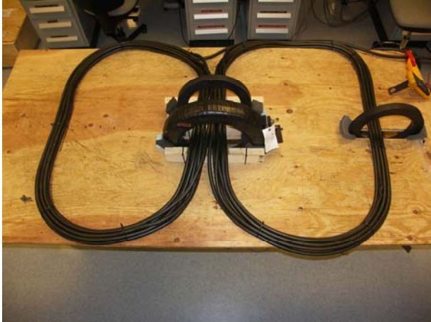
Figure 2 – Grand Coulee Powerplant - CT Calibration (Fourteen loops of cable pass through both the larger plant CT and smaller standard CT located in the middle of the table.)
