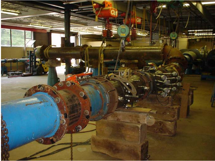
Figure 4: Example of Calibration with Meter in Close Proximity to Non-Planar Coupled Upstream Elbows
