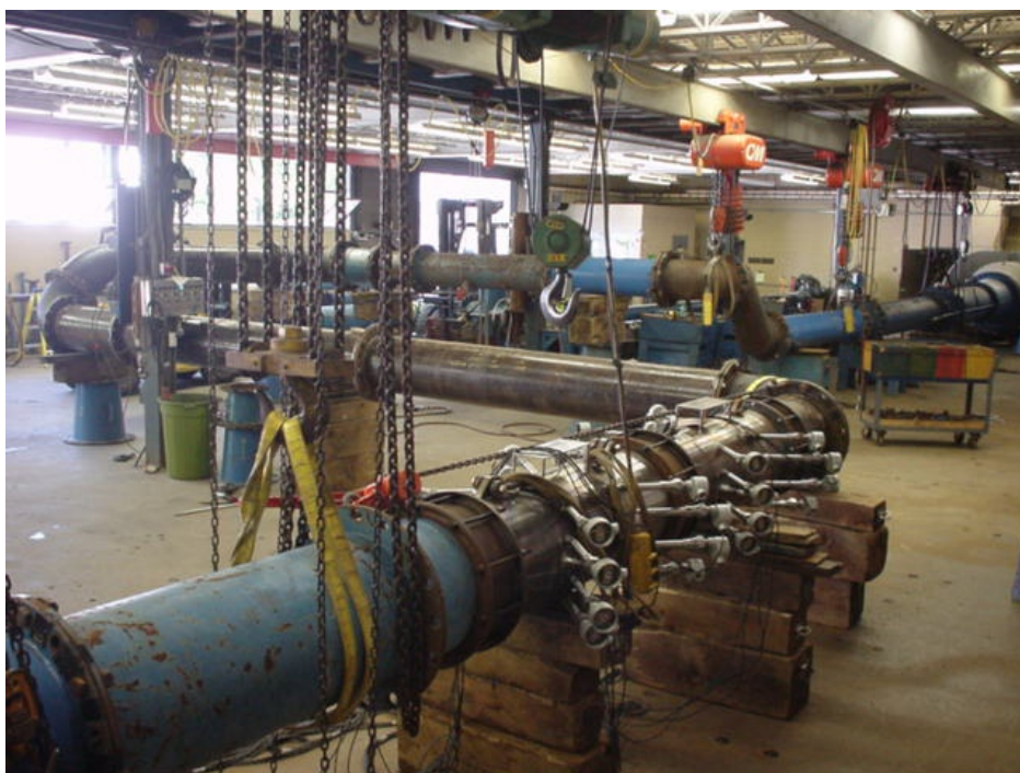
Figure 3: Example of Calibration with Non-Planar Model Components with Meter in Close Proximity to Upstream Elbow (Two meters shown)
