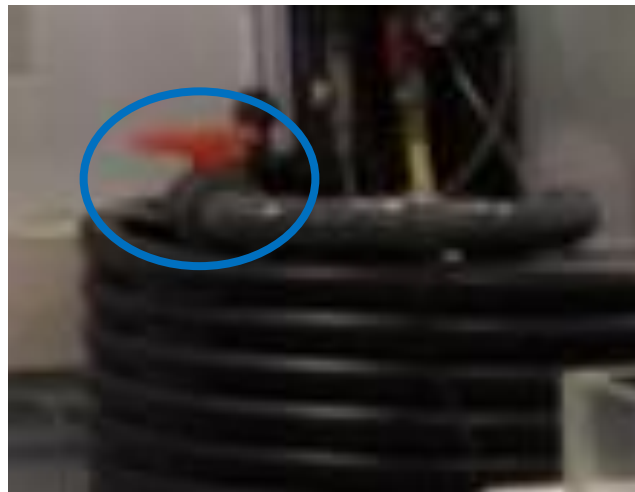
Fig. 3 shows V1 valve, which is a spherical valve used to start the flow in the circuit. It is installed at the output of the upstream reservoir.
