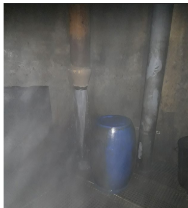
Figure 6: Dewatering room conditions for shaft seal leakage measurement
