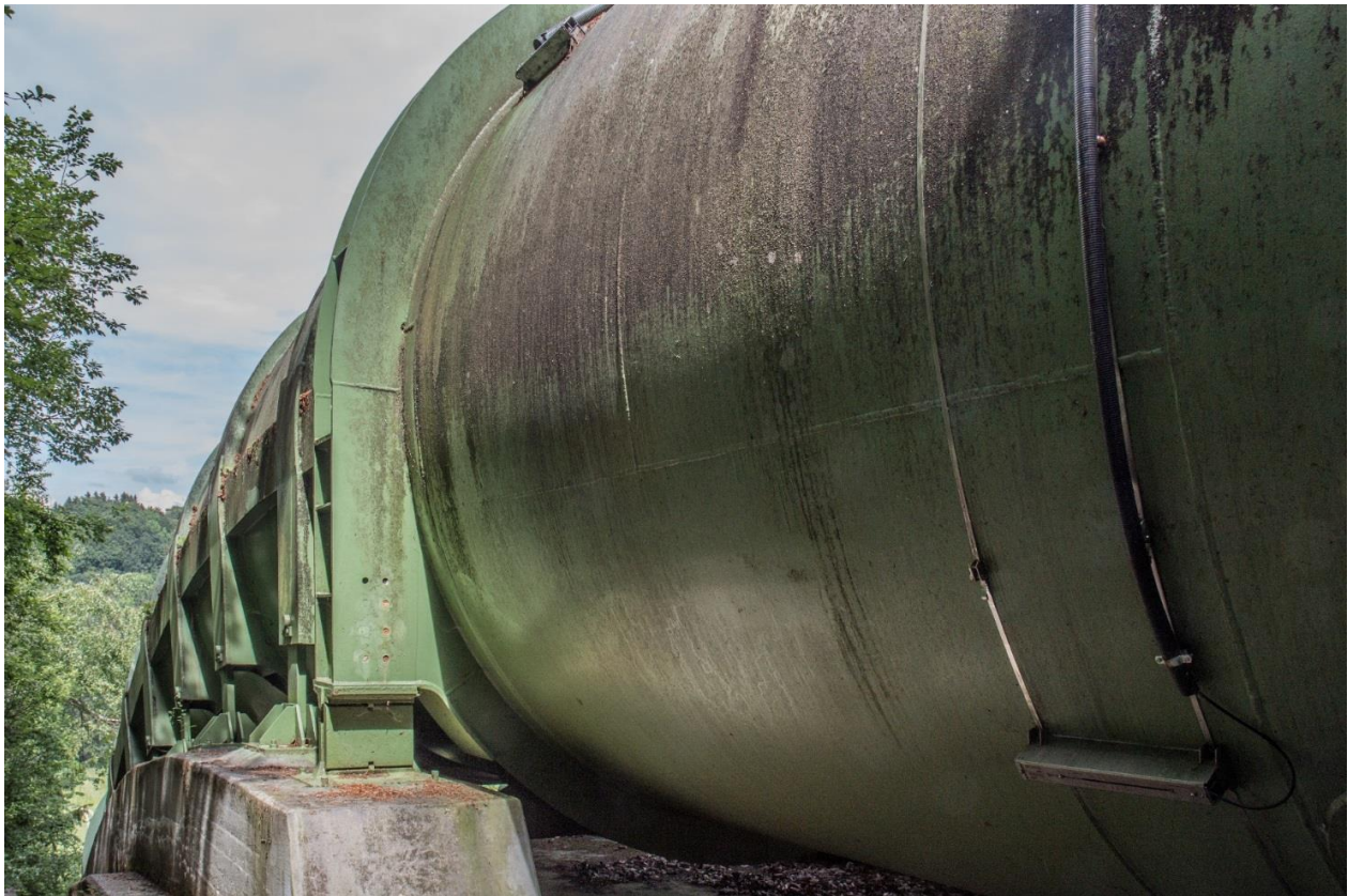
Fig. 6 – Example of a non-intrusive ultrasonic flow measurement installation by FLEXIM on a penstock of a pumped storage plant, 2-channel with 1 sound path each
