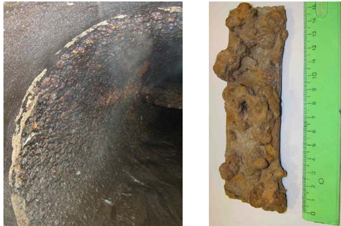
Fig. 1 – Penstock inside incrustation
