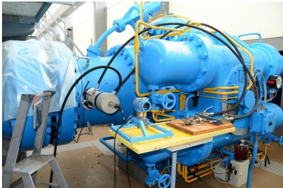
Figure 9: Instrumentation for thermodynamic method on the inlet side
